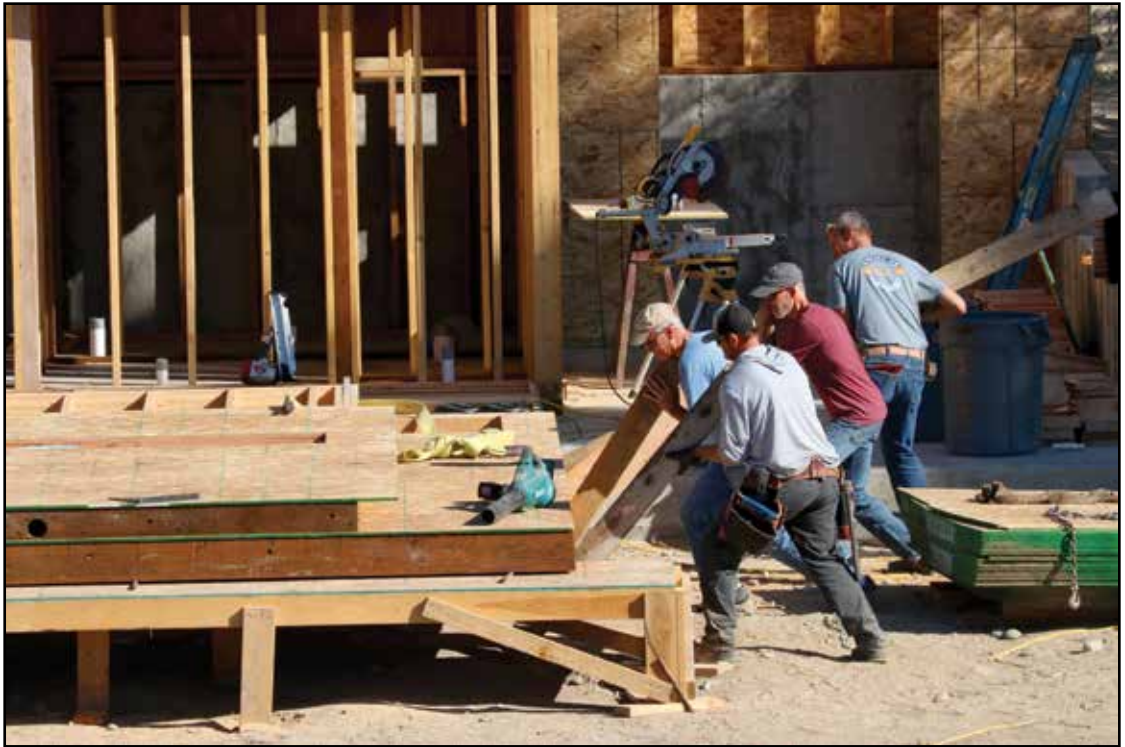
Workers erect two new homes in Eureka near Timbers Lodge in October 2022.
